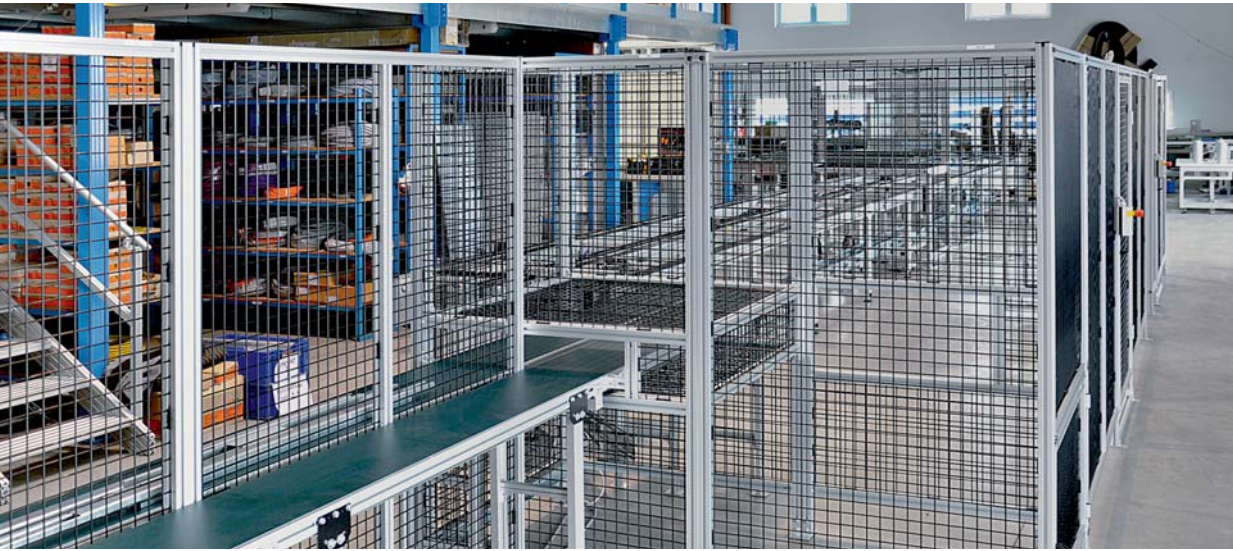
Guarding with welded grids (partition method) for tray transport system
